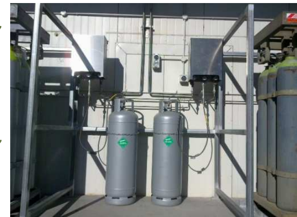
Typical Gas Installation showing two BSL Gas-Mix FW Panels in operation.
