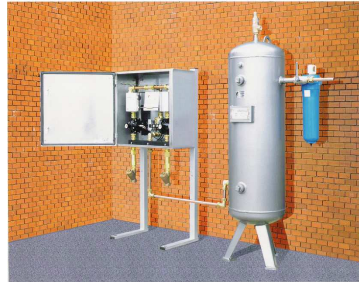
Gas-Mix HF assembly, 500 nm 3 /hr with associated buffer tank and filters.
