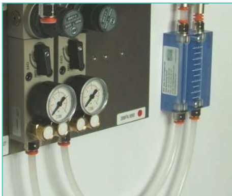
In Line Leak Indicator on the outlet of a BSL Cellar-Mix Beer Dispense Panel.
